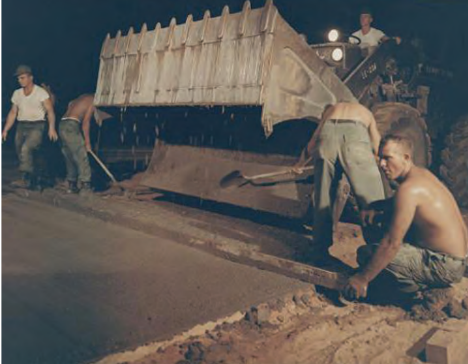
Because of high daytime temperatures, crews pave concrete pads for buildings at Cam Ranh Bay at night.
